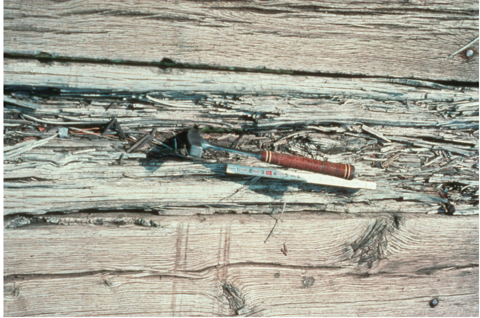
Figure 2.1.24 Weathering on Timber Deck
