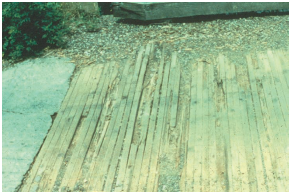
Figure 2.1.21 Wear of a Timber Deck
