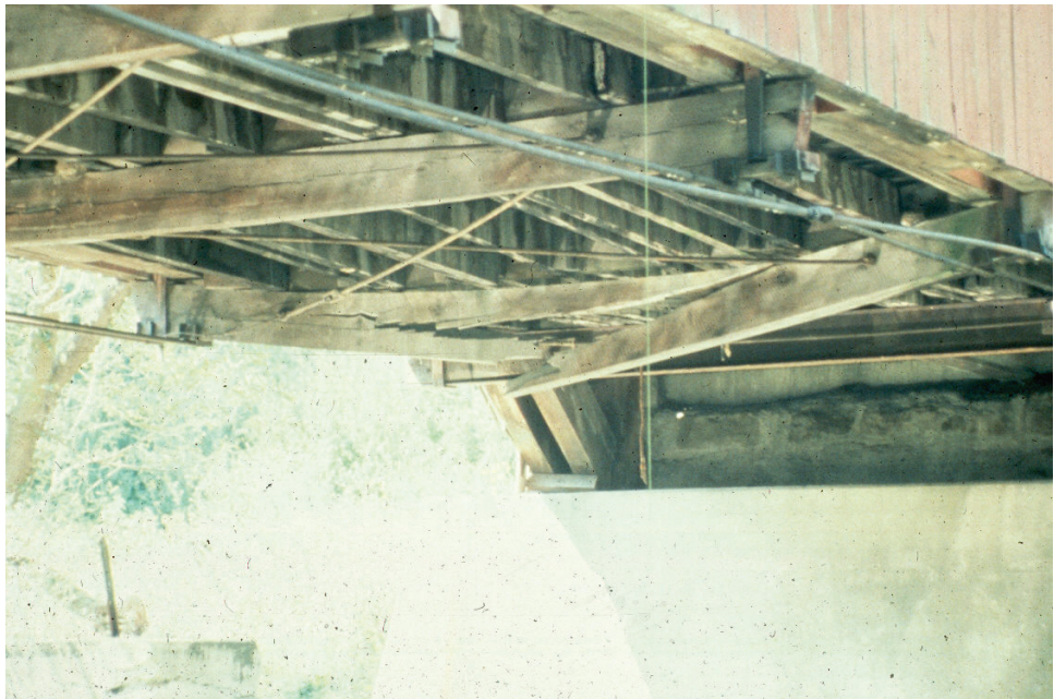
Figure 2.1.23 Failed Timber Floor Beam due to Excessive Bending Moment
