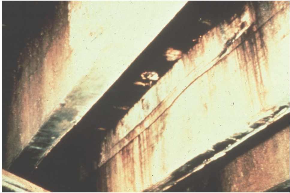
Figure 2.1.22 Horizontal Shear Failure in Timber Member
